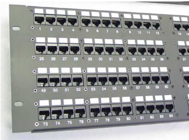
Network Patch Panel
